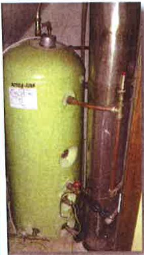
19.21 Insulated hot water cylinder.
